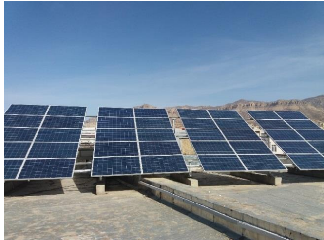
Fig. 1. PV plant under examination.
